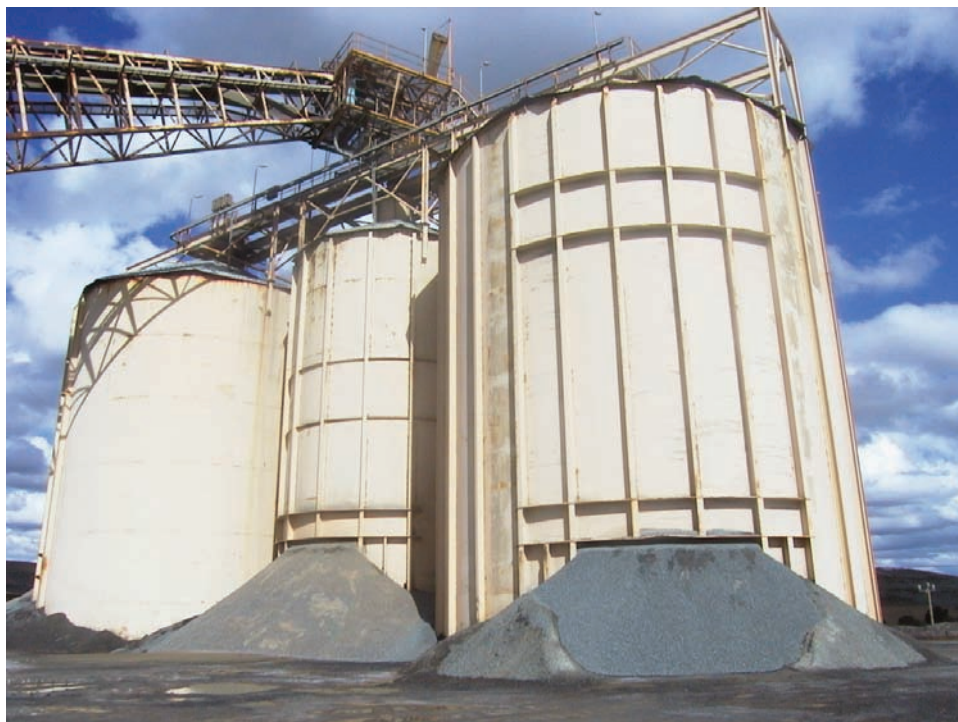
FIG 5 - Fine ore bins, Cornishman Joint Venture (on right).
