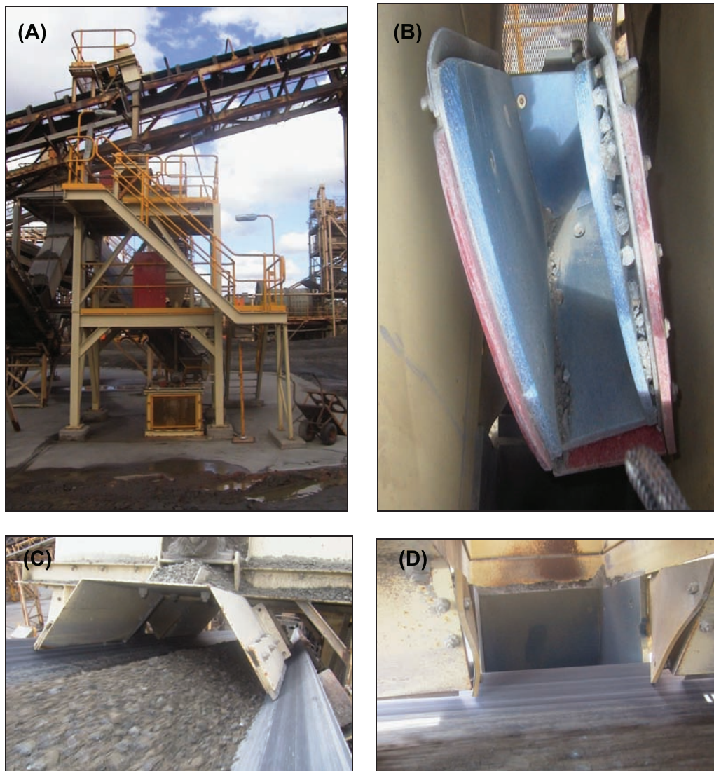
FIG 3 - (A) Sample plant overview; (B) primary cutter; (C) primary sample point; and (D) primary sample transfer chute.
